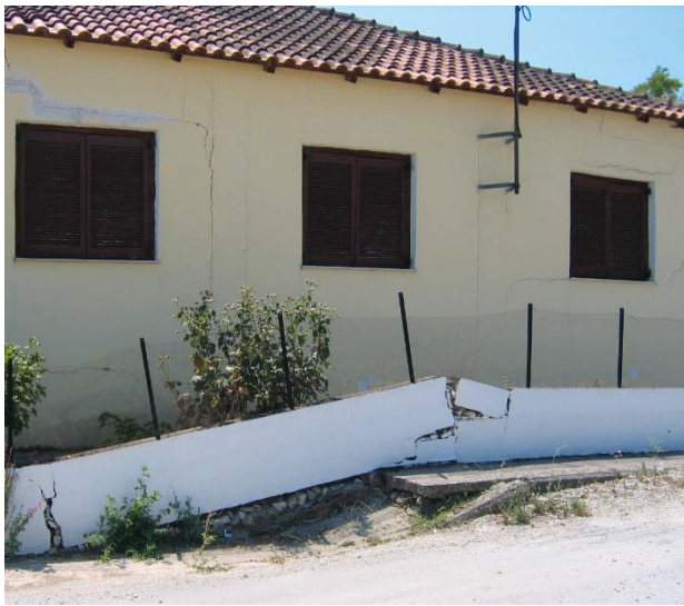
Figure 1 Damage caused to the building due to the ground fissure.
