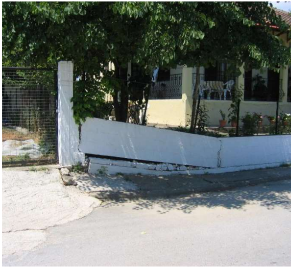
Figure 1: The impact of ground fissure on the structural integrity of the building.
