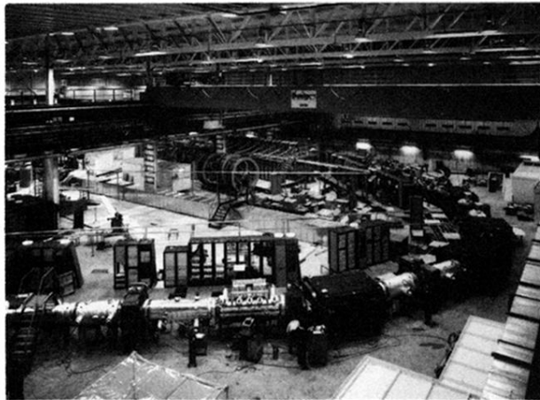
FIG. 15. View of the Antiproton Accumulator before it was covered by concrete slabs. The silvered material around the vacuum tanks is insulation, needed because everything may be heated to 300^{\circ} to obtain ultrahigh vacuum. The transmission lines crossing the ring and carrying the cooling signals may be seen.
