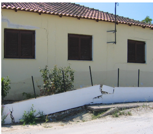
Figure 1 Damage caused to the building due to the ground fissure.
