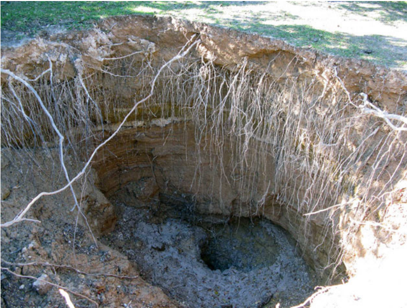
Fig. 3.17 6–8 m deep and 8 m in diameter “doline-type” hole next to the rupture of November 2011. The filling was washed away through a drainage
